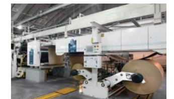
Printing Factory, Malta, AHU
